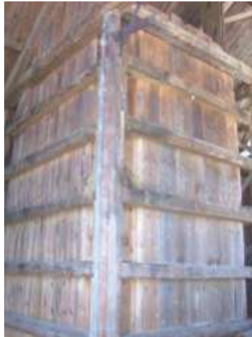
Square Indoor silo
